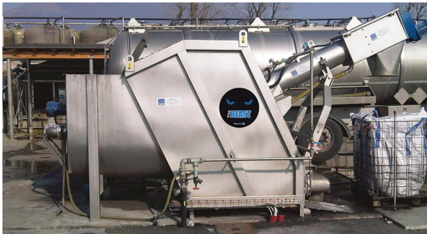
Figure 30: Picture of Prefabricated Mechanical Screens
