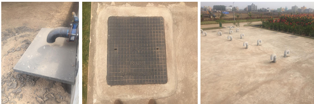
Figure 37: (A) Splash plate (B) Manhole cover with bituminous coat (C) Vent pipe installation
