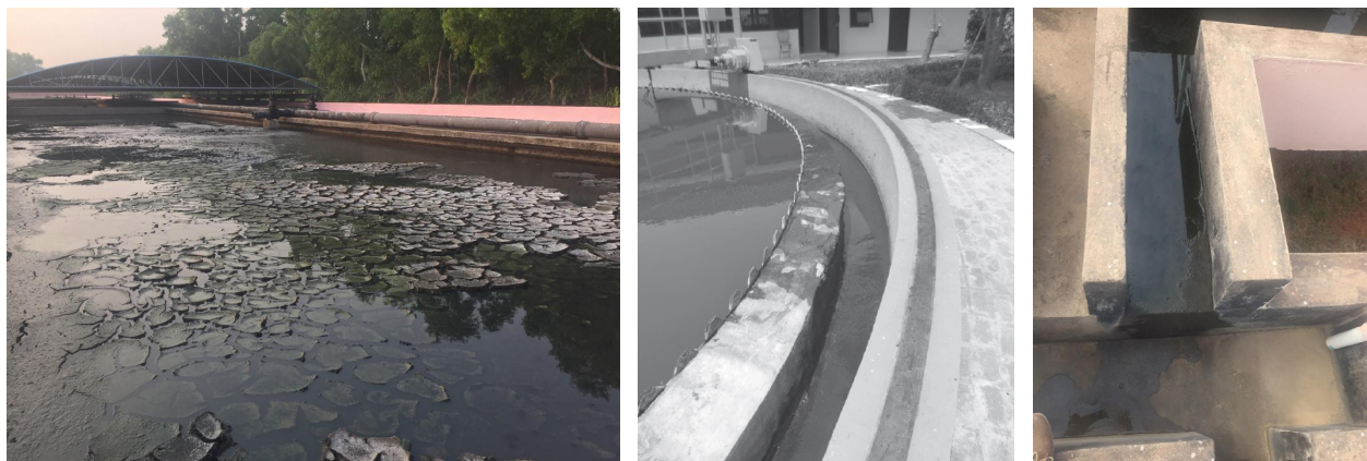
Figure 36:( A) Poor distribution of sludge over drying bed (B) Unbalanced flow from clarifier (C) Poor slopes in the channel
