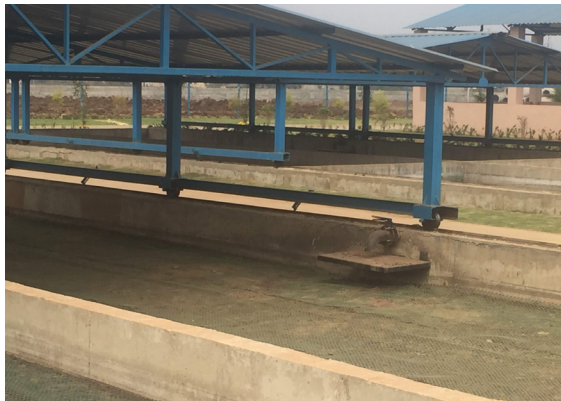
Figure 50: Easy Access To Valves From Outside Of The Bed
